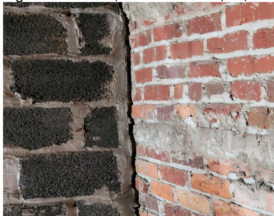
Figure 4. Wall separation and improper repairs.
