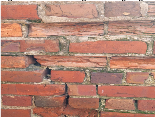
Figure 3. Deteriorating brick on garage.
