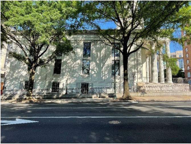
Figure 5. View of the east elevation of St. Paul's Episcopal Church, along North 9 th Street.
