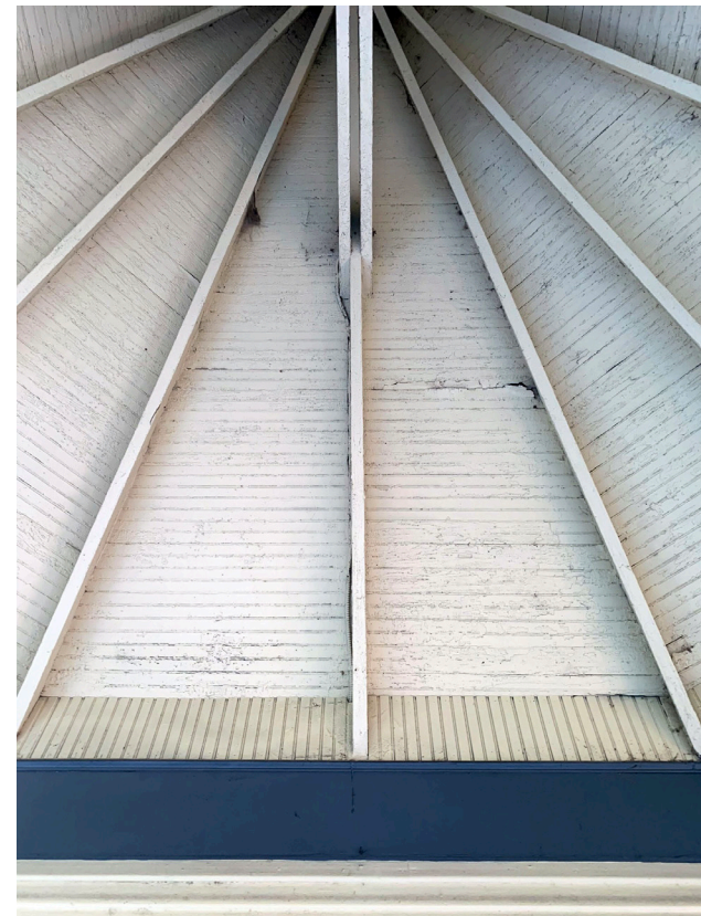
Peeling paint gazebo roof decking
