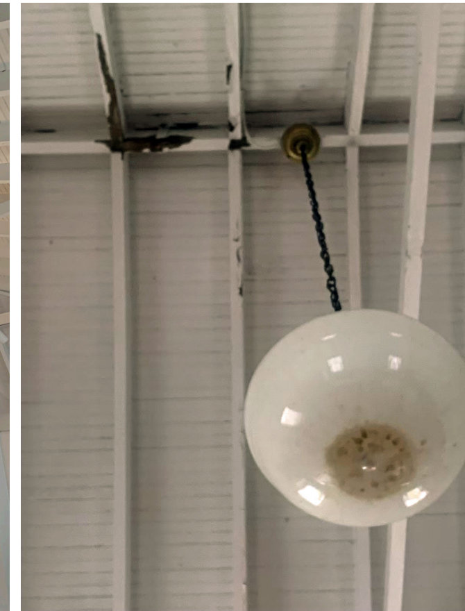
Interior image showing water damage
