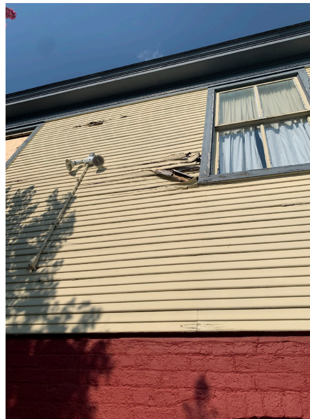
Damage to exterior siding
