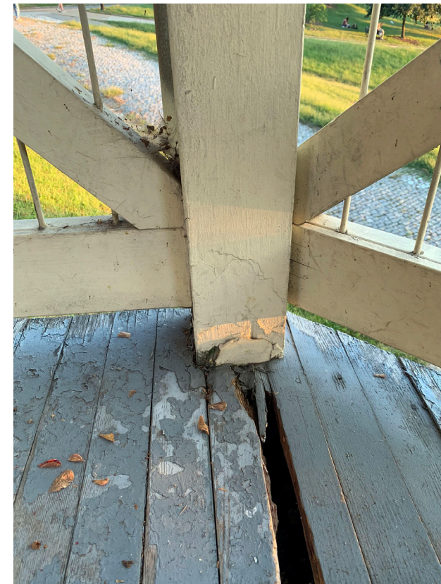
Damage to post and decking prior to Phase B
