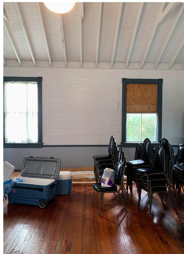
Interior detail showing window damage
