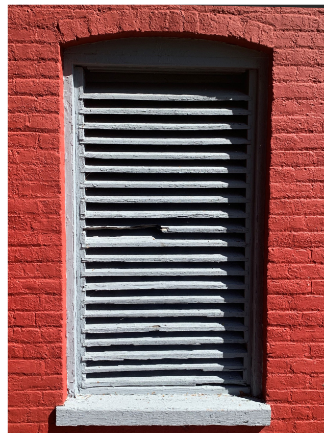
Example of damage to exterior louver
