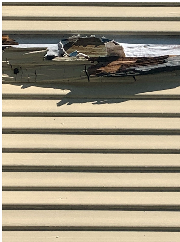
Example of damage to exterior siding
