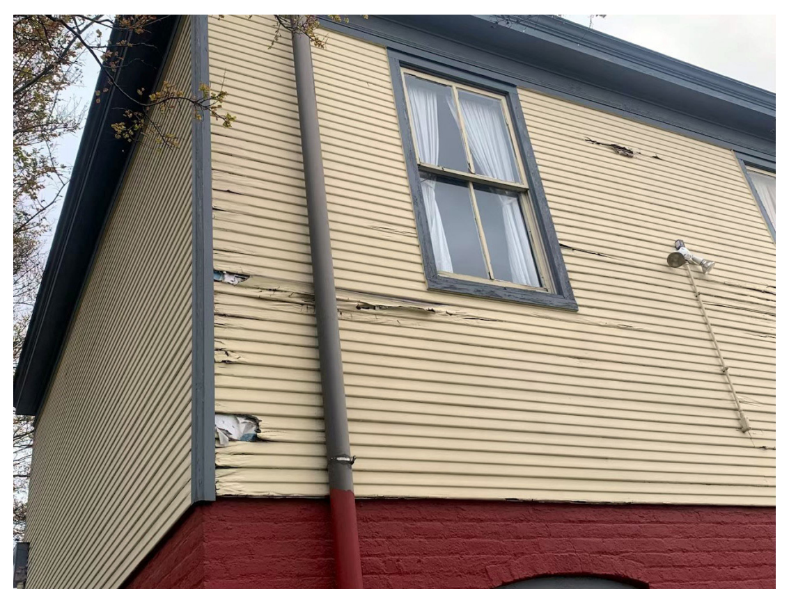
exterior detail of damage (image taken before window sash fell out)
