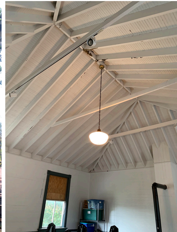
Interior image showing water damage
