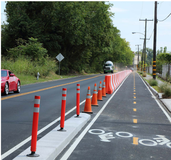
Figure 14. Federal and State funding priorities dictate which projects a local government can build. Major bicycle and pedestrian infrastructure, like the Virginia Capital Trail, can take years to complete due to scarcity of funds for non-automobile projects.
