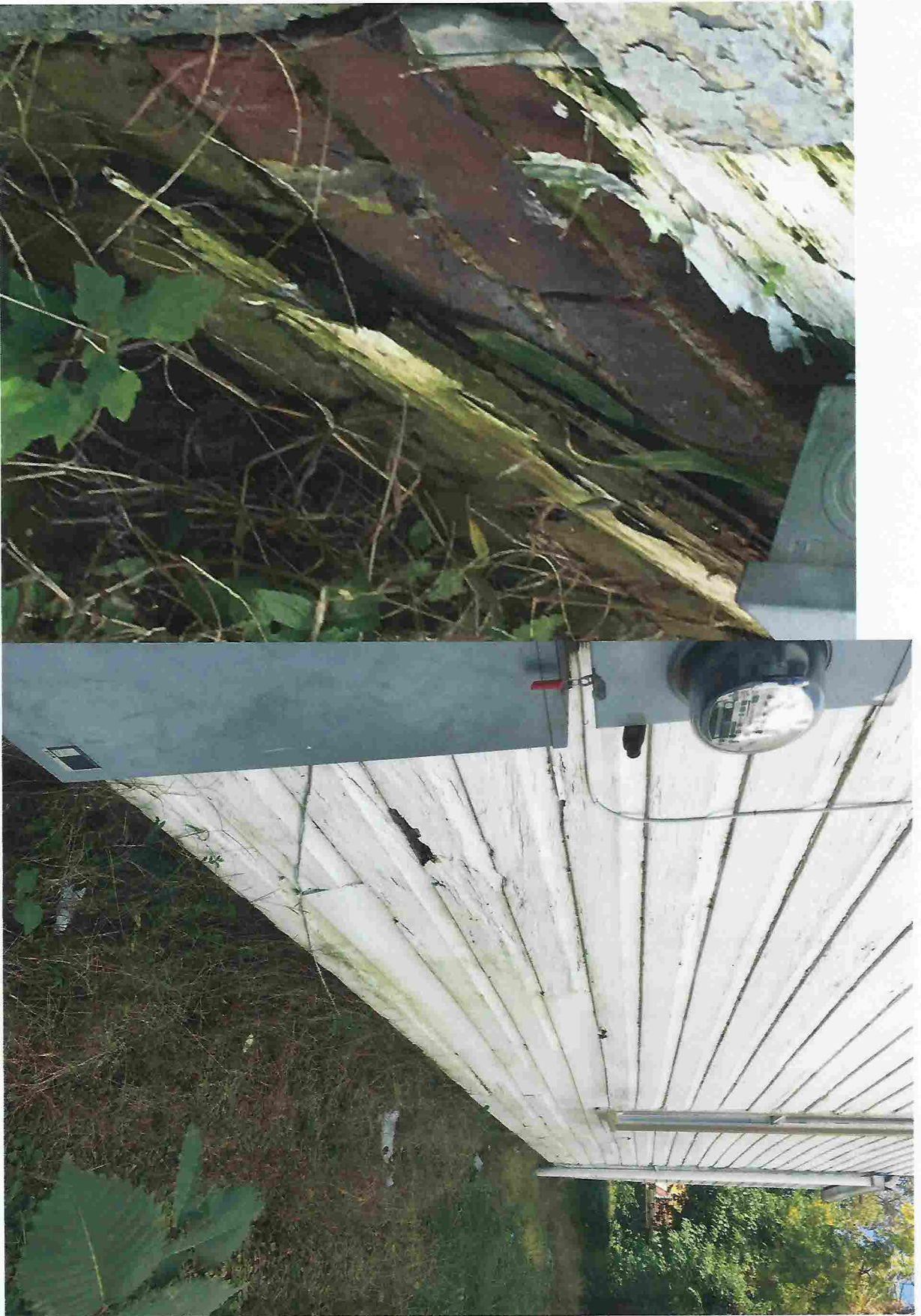
Wood siding has major damage due to water issues and age.
