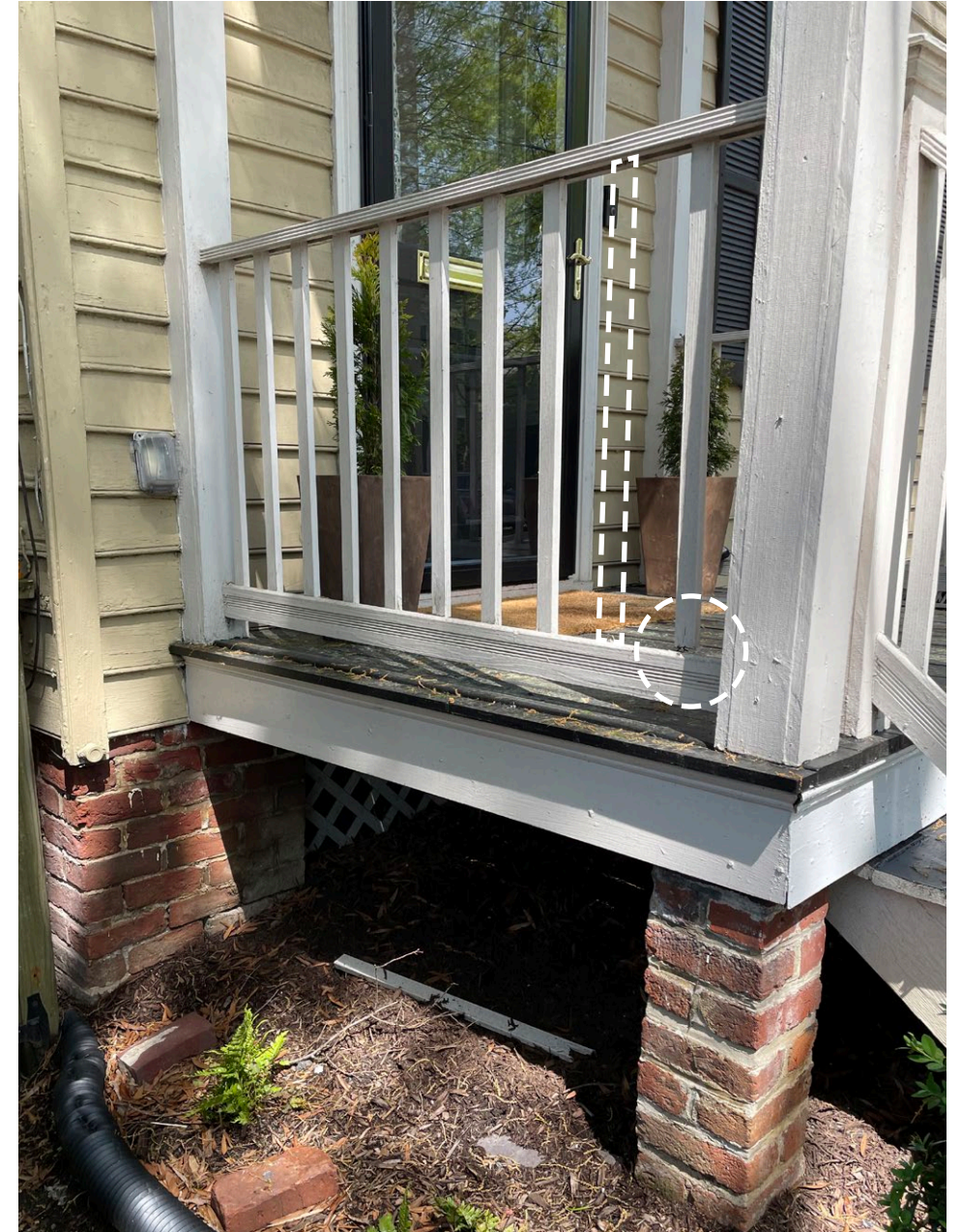
EXISTING FRONT PORCH SHOWING TYPICAL PICKETS TO BE REPAIRED / REPLACED IN KIND
