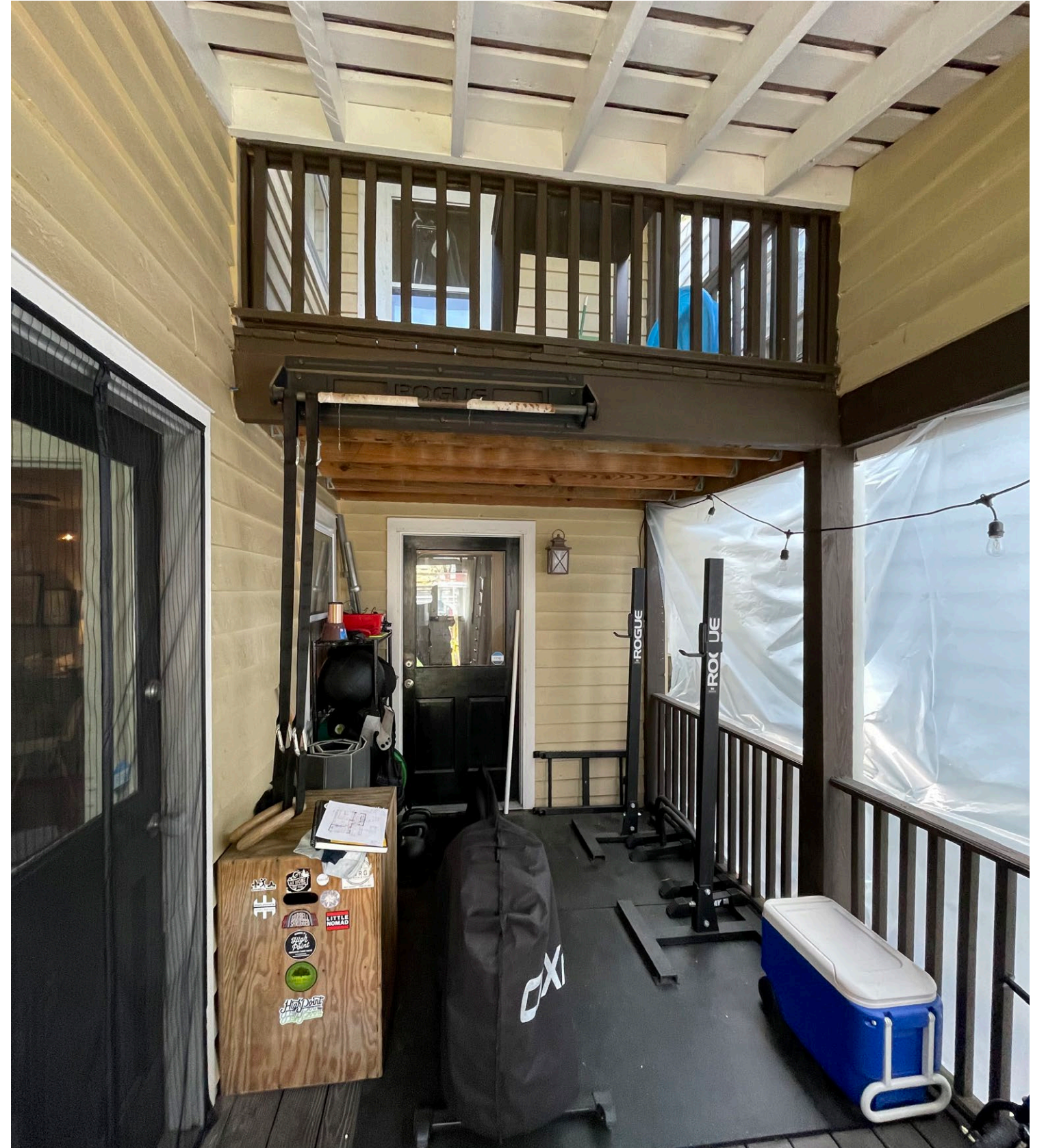
EXISTING NON-ORIGINAL SIDE PORCH W/ CONTEMPORARY FRAMING ELEMENTS AND NON-HISTORIC SIDING AND TRIM ELEMENTS
