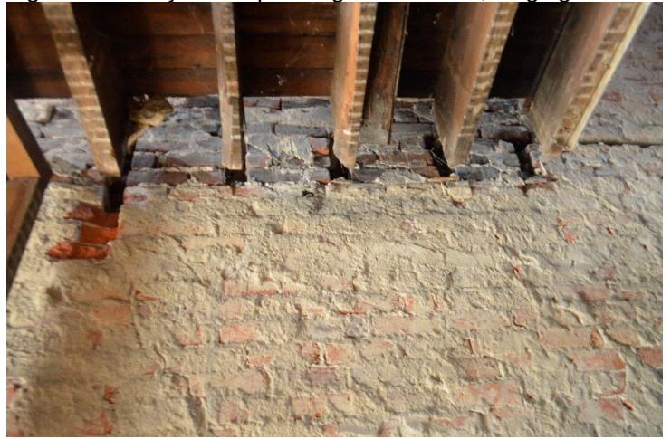
Figure 4. Floor joists separating from interior, bulging wall.
