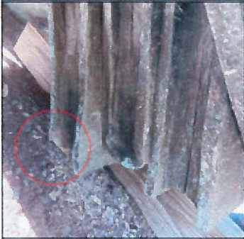
Book corner damage
