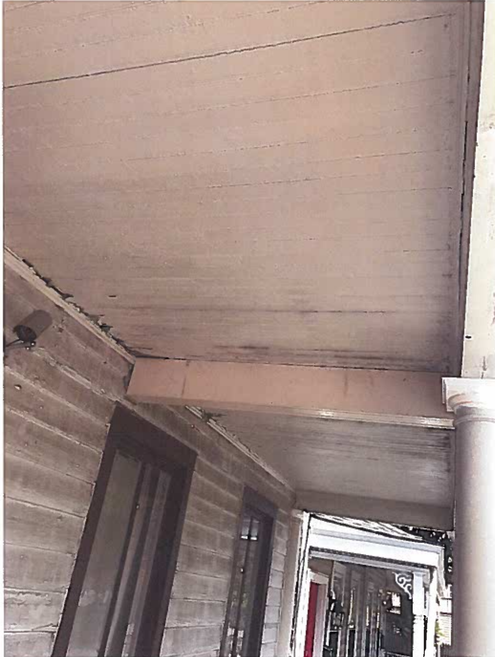
Exterior Front Porch Ceiling: Ceiling to be maintained and repaired/painted White.
