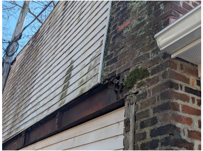
Figure 7: deterioration of the historic brick
