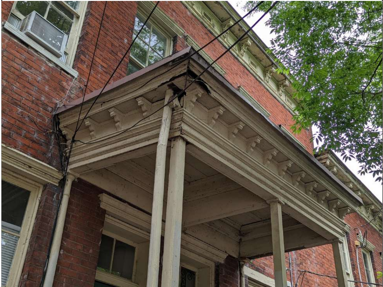
FRONT PORCH TO BE REPAIRED
