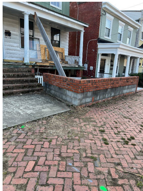
Figure 2. Showing condition of brick retaining wall
