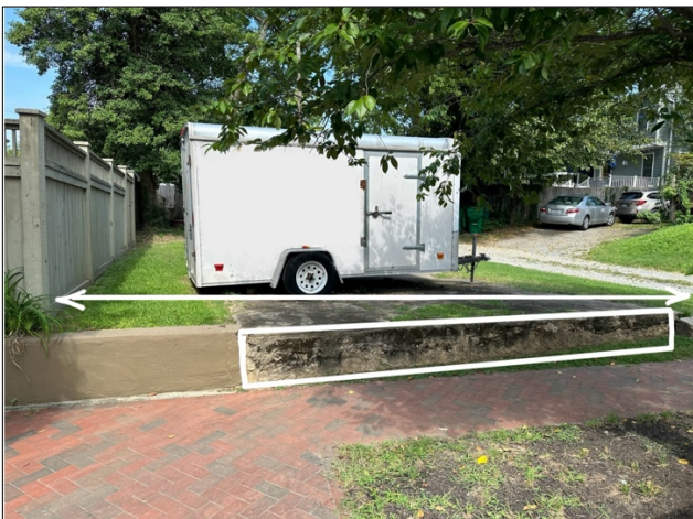
Fence line to be extended. Retaining wall to be repaired. New stair and fence (match existing) to be constructed.
