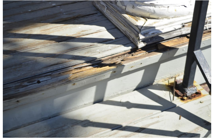
Figure 10. View of the southeast column and further deterioration of the deck boards.
