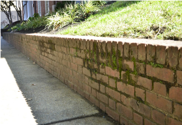
Figure 7. View of the brick wall on the west side of the property. The wall will be repaired and retained after the new staircase is added to the wall.
