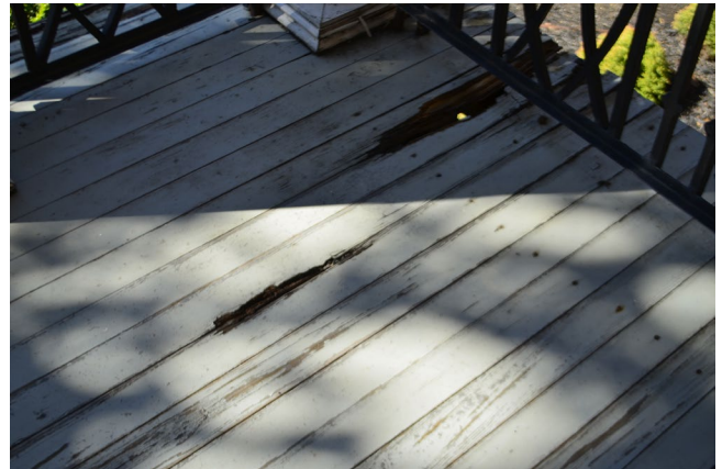
Figure 8. View of deteriorated wooden board on the porch facing Grace Street. This porch will be repaired with in-kind materials.
