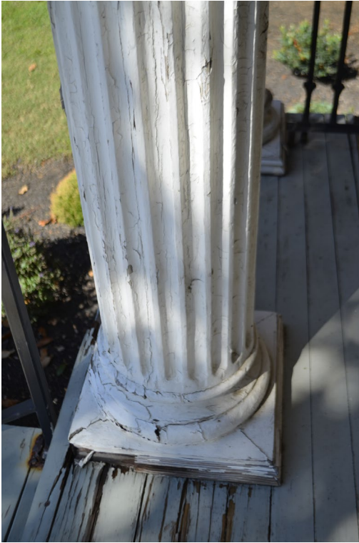
Figure 9. View of deteriorated wooden deck boards and a deterioration at the bottom of the southwest column. The owner plans to repair the deck boards and column with in-kind materials.
