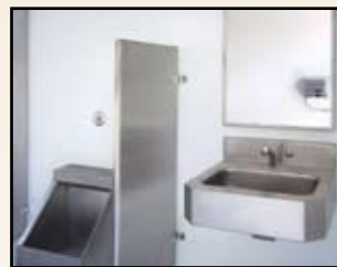
Stainless Steel Fixtures
