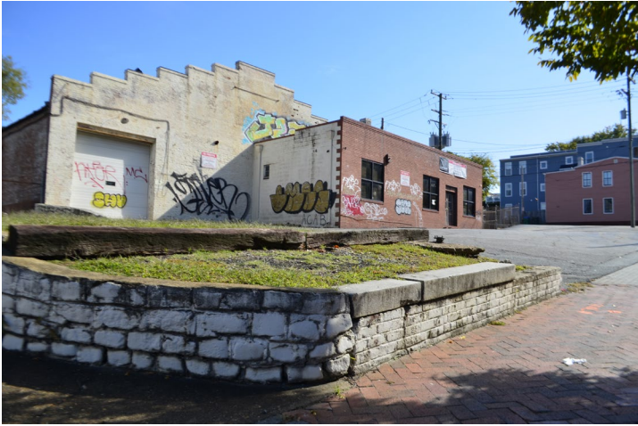
Figure 13. Masonry and brick wall at the southwest corner of the site. This wall will be replaced with a new, low brick wall.
