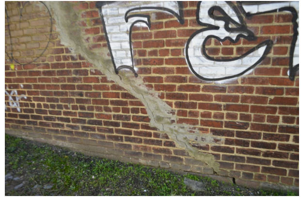
Figure 8. View of deteriorated masonry on the north side of the building.
