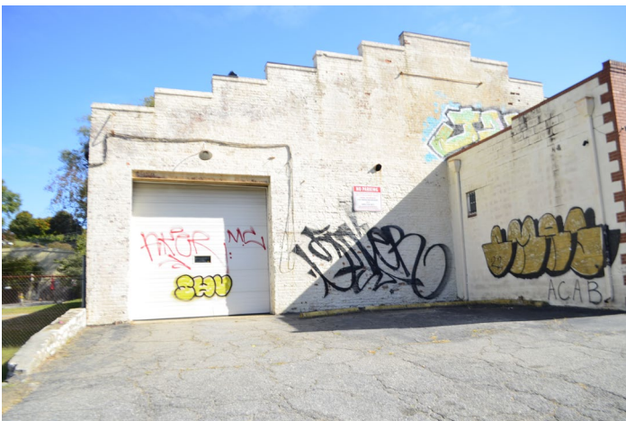
Figure 9. View of the painted masonry on the south side of the building. This side will be cleaned, the graffiti removed and repainted.
