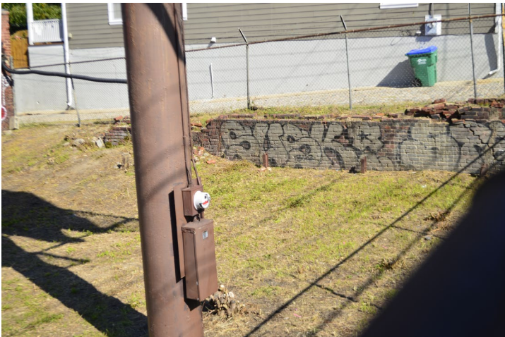
Figure 15. View of the historic wall at the northeast corner of the lot. The historic masonry retaining wall will be maintained and repaired in kind. Failing sections of the brick wall will be rebuilt.
