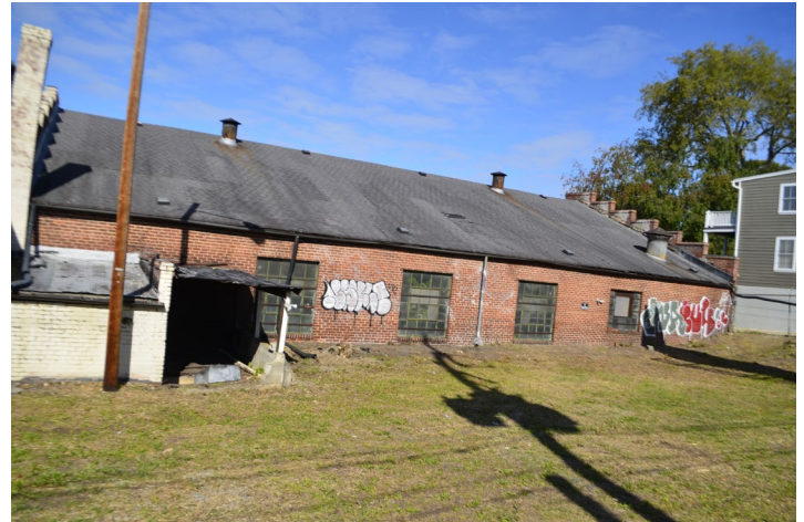
Figure 10. View of the east side of the building. The boiler room can be seen on the left side of the photograph. The open, shed section, north of the boiler room will be removed. The steel windows on the west and east sides will be kept in place and repaired.
