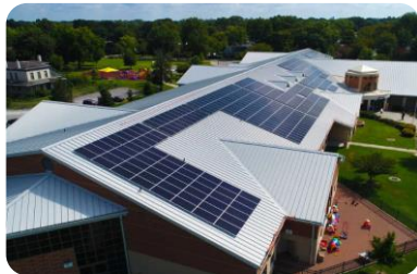
SSF installed rooftop solar through a PPA on J.H. Blackwell Elementary School, 300 E 15th St, Richmond, VA 23224
