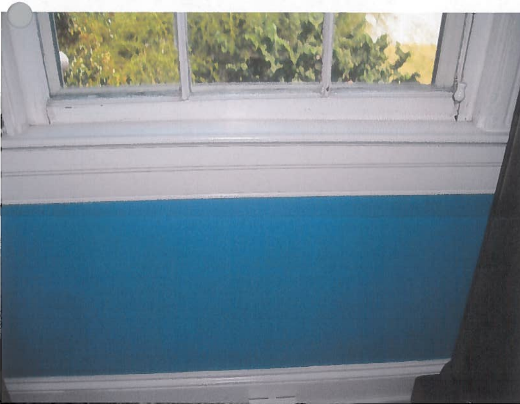
Figure 7: The window sill is level but note the how the window itself is tilted up on the right side.
