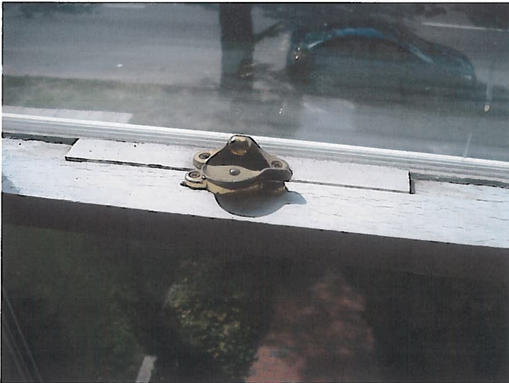
Figure 8: this is also one of the windows that needs to be shimmed to keep out the cold air in winter.
