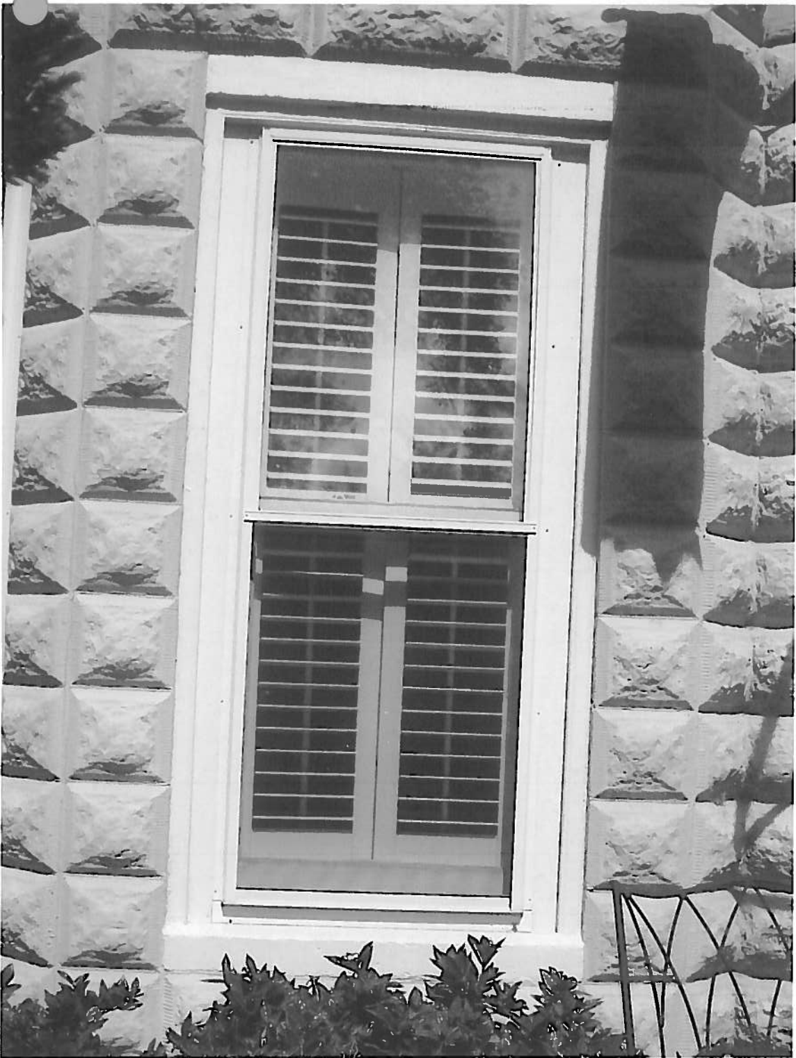
Figure 6: Close up of existing front window.
