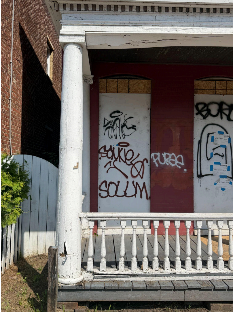
18. Railings to be repaired and base plate to be replaced in kind. Missing pickets to be installed with in kind pickets and others repaired as needed.
