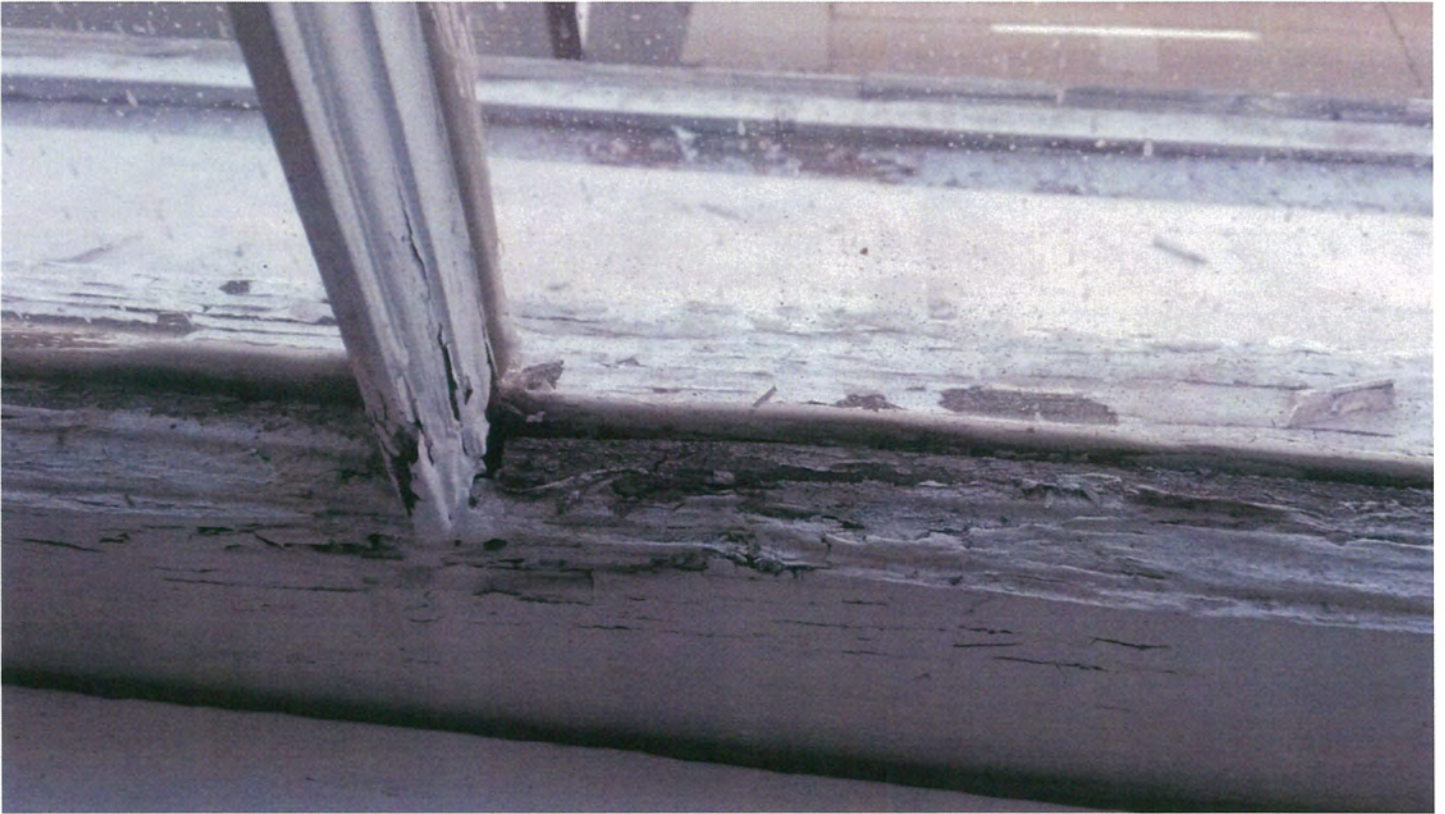
Dry rot and muntin no longer connects to sash.
