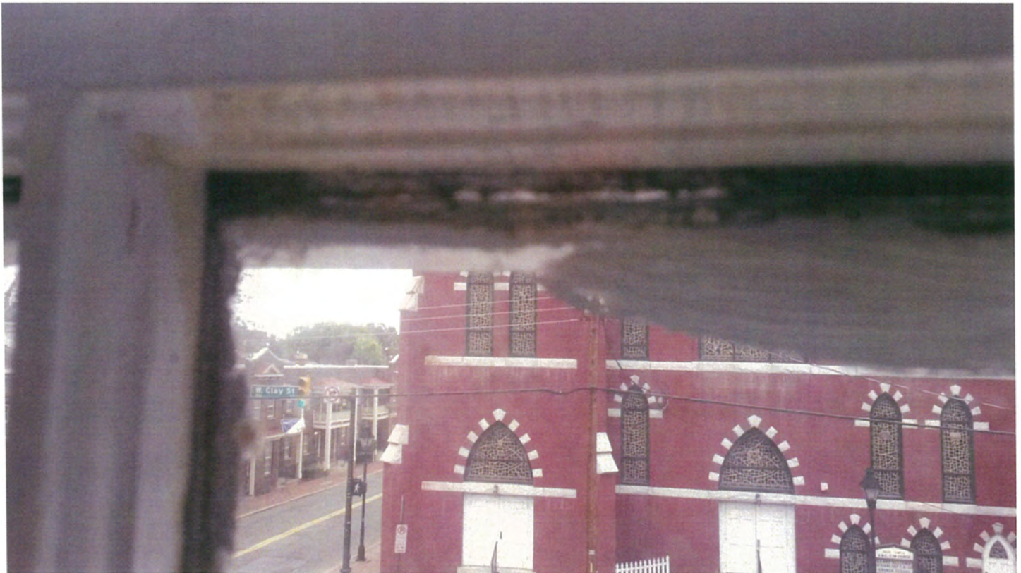
Window glazing broken and detached from muntin.
