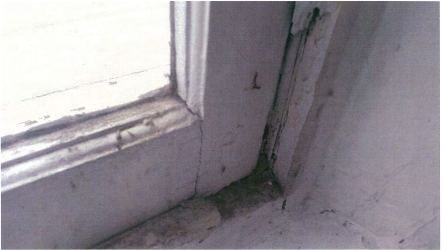
Rotted and Broken jams.
