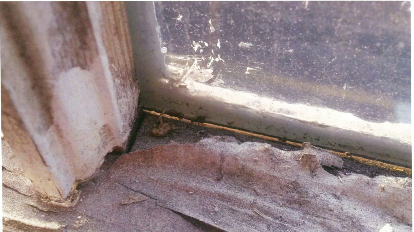
Muntin no longer connects to sash. Evidence of rot to sill.
