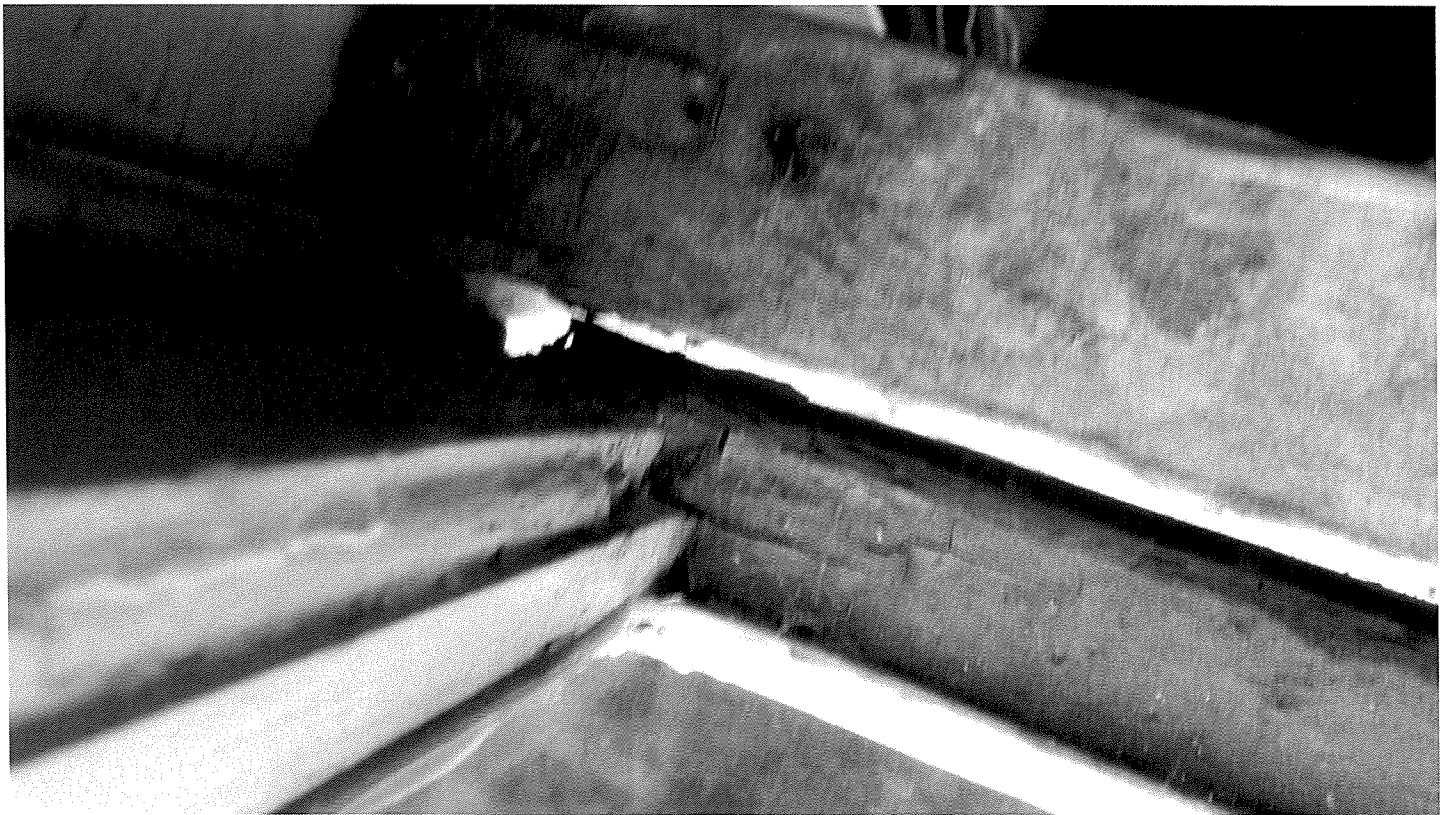
Exterior window sash rotted.
