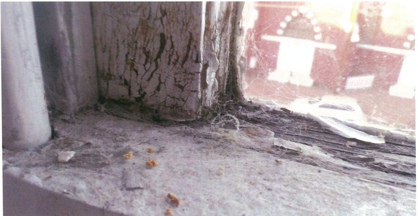
Wood rot and what appears to be mold or fungus.
