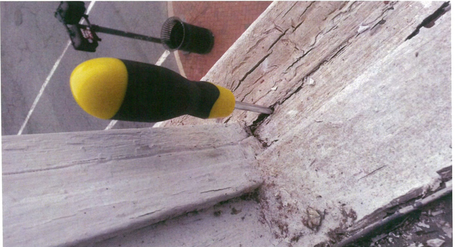
Sill wood rot.
