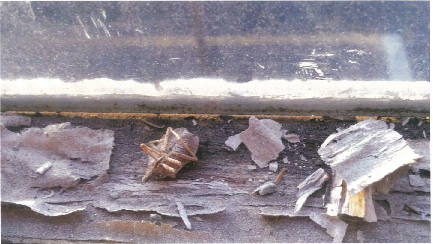
Glazing no longer connects.
