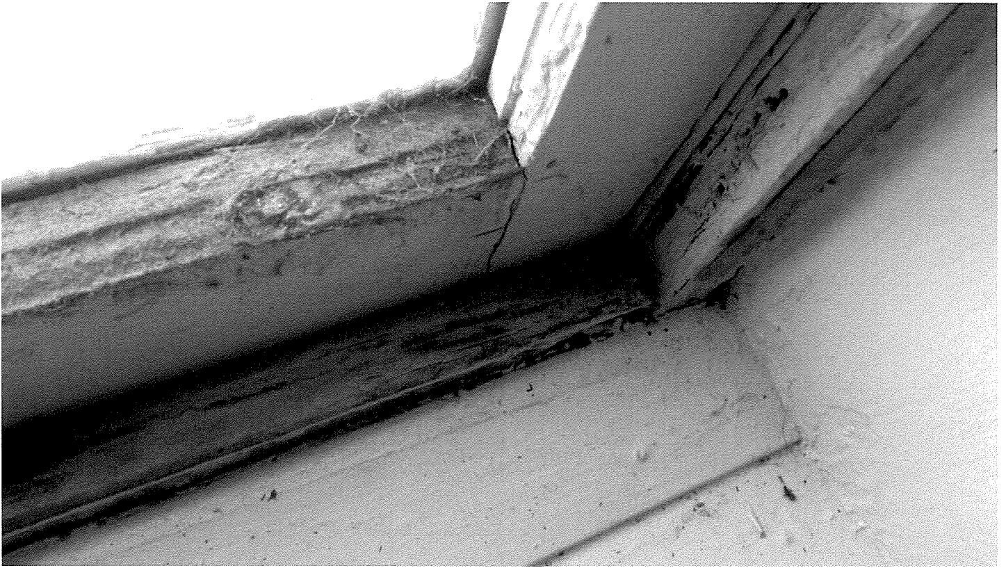
Interior dry rot.
