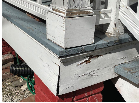
Figure 2. 510 North 29 th Street Existing Conditions. Deteriorating column base, railings, and skirt board.
