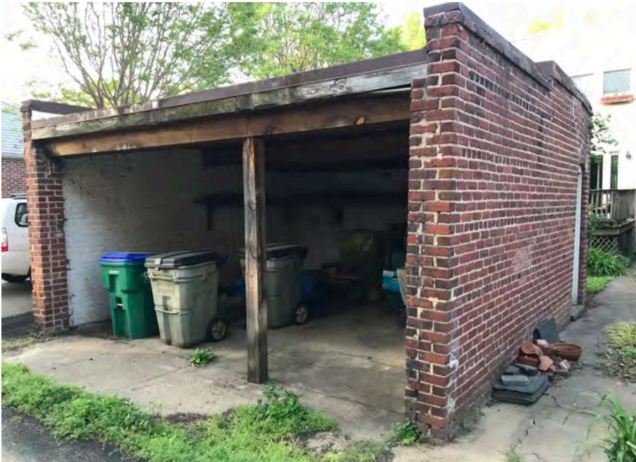
South-East view from alley showing cracked and leaning wall on right and deteriorating concrete slab
