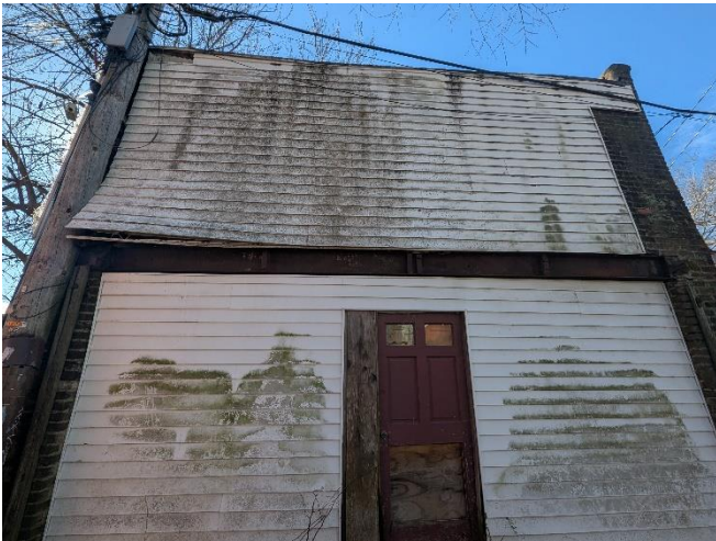
Figure 10: siding appears to have been used to replace deteriorated brick
