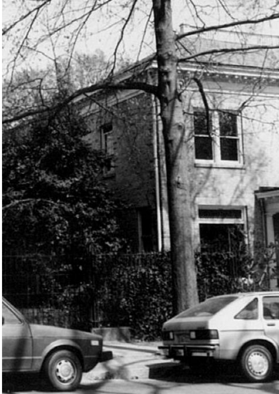
1208 W. Franklin Street, 1969 or 1970, showing the missing roof balustrade
