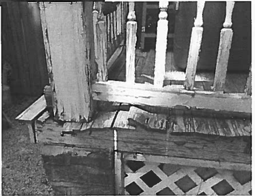
WOOD ROT AND CRUMBLING FLOOR, RAILINGS AND POSTS
