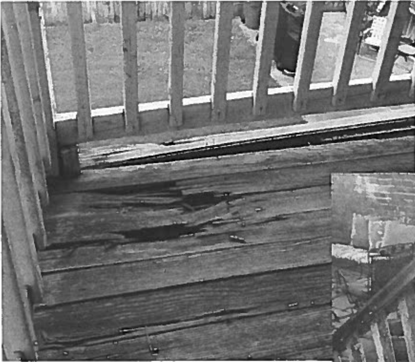
HOLES IN FLOORS UPSTAIRS AND DOWN
