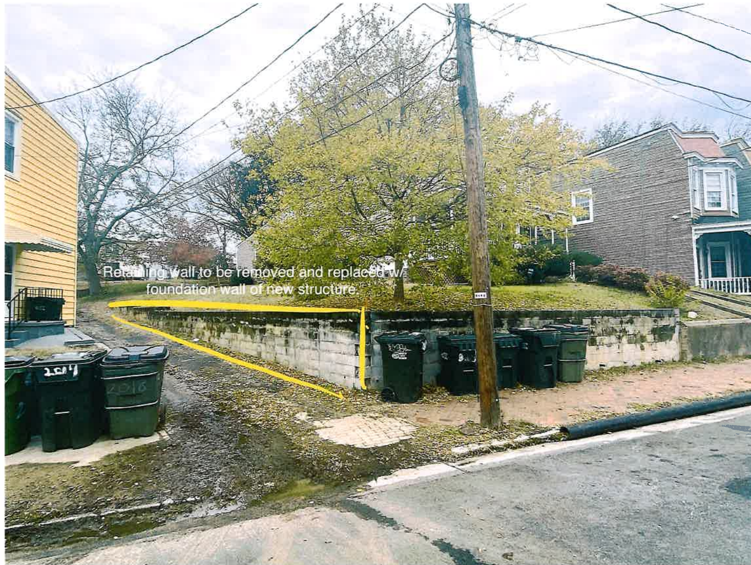
Existing retaining wall on the south side of parcel to be removed and replaced by the foundation of the proposed duplex.
