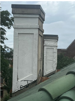
Figures 4. Westernmost, intact chineys.
