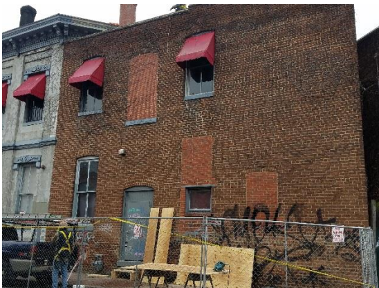
Figure 3. 200 West Marshall Street, rear section and location of proposed fire escape stairs.
