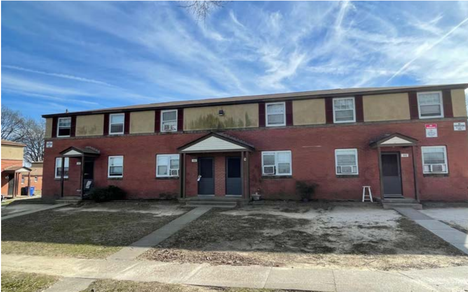
1412-1418 Bruce Street in Hillside Court. This shows the deteriorating exterior of public housing.
