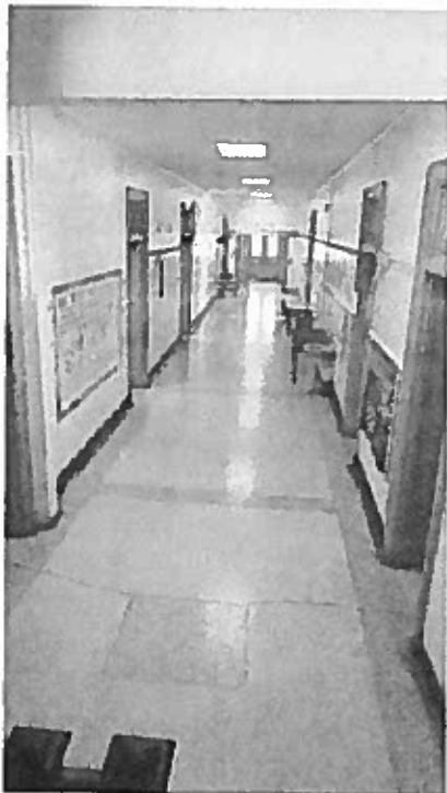
Figure 10. Cracking terrazzo floors, 1922 section.
