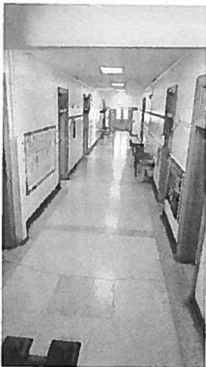
Figure 10. Cracking terrazzo floors, 1922 section
