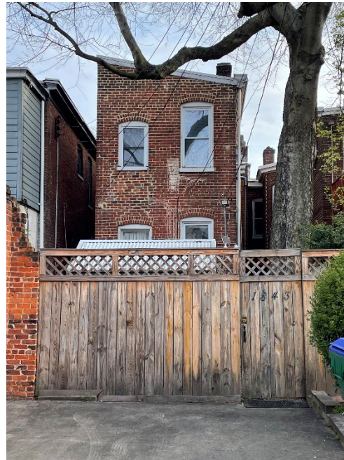
Figure 2. View of the south elevation of 1843 West Grace Street, along the public alley.
