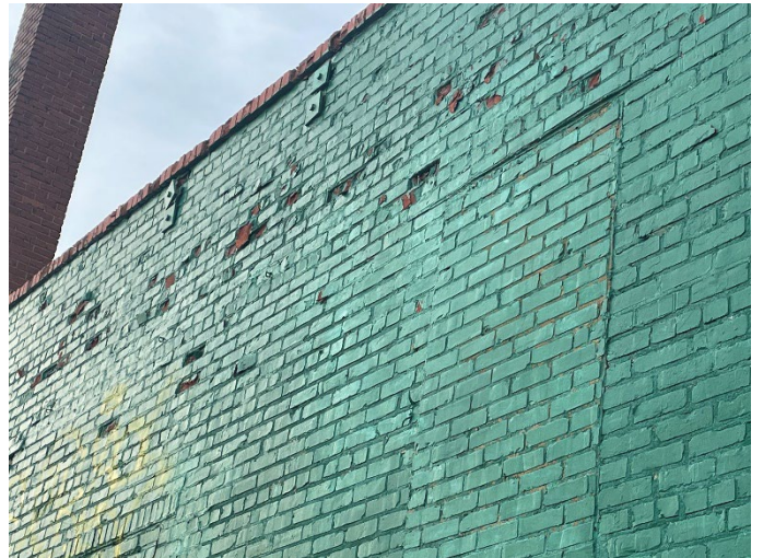
Figure 8. Brick Spalling example.
