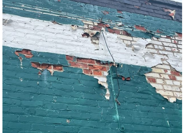
Figure 6. Brick Spalling & Possible improper repointing example.
