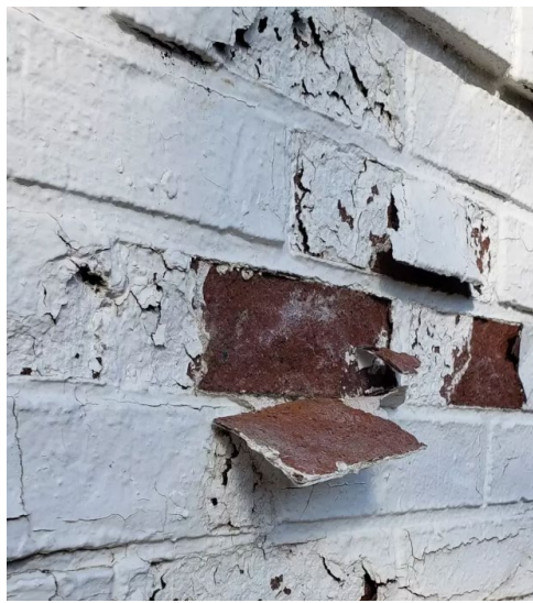
Figure 4. Brick Spalling example
