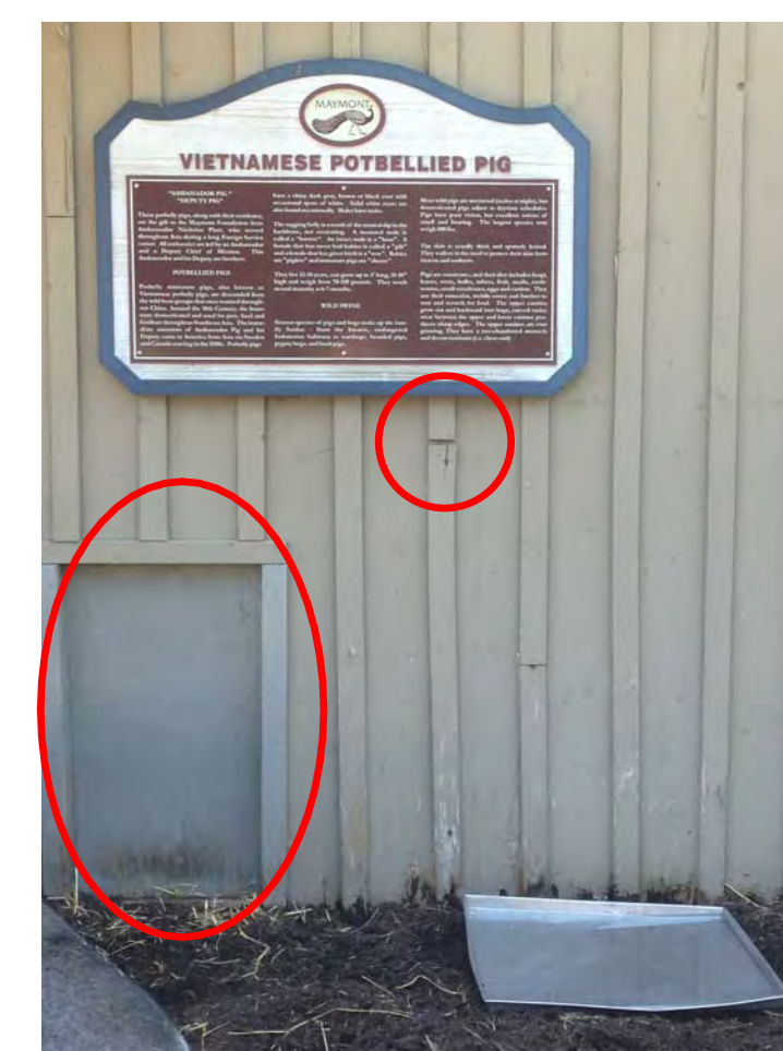
4. REMOVE ANIMAL ACCESS DOOR ON NORTH BARN WALL. PATCH WALL AND SIDING. REPAIR BOARD AND BATTEN WHERE GAPS > 1/2". REPAINT. TYP. FOR ALL BOARD AND BATTEN SIDING.
