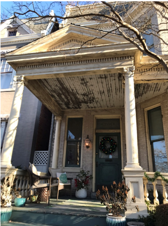
Figure 3. Front porch disrepair
