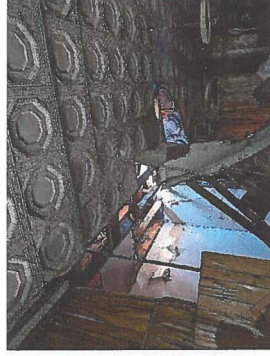
EXISTING INTERIOR 2ND FLOOR ROOF COLLAPSE
