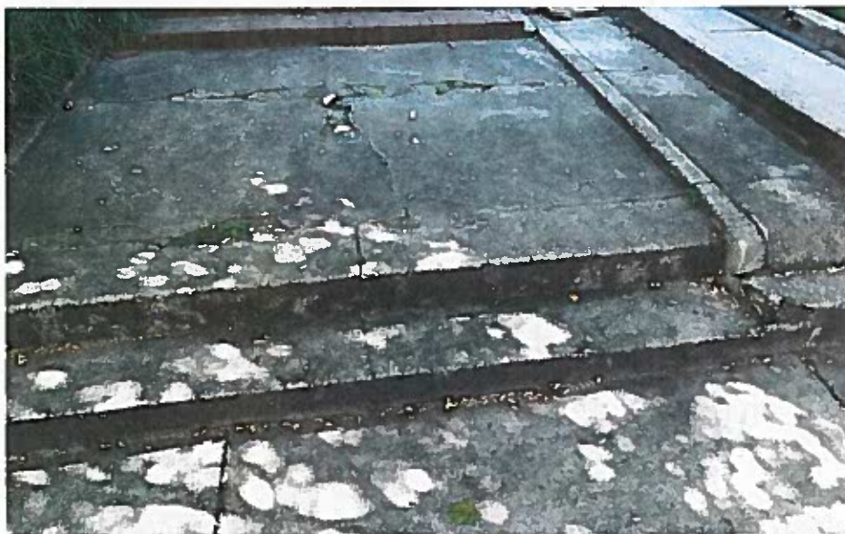
Current Condition of walkway.
