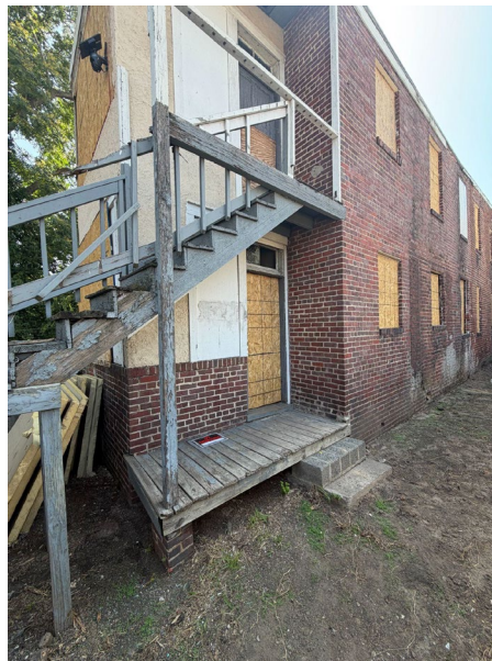
Figure 4. Existing condition of south elevation of 606 North 1st Street, including deteriorated decking and doors on the rear sleeping porch enclosure.
