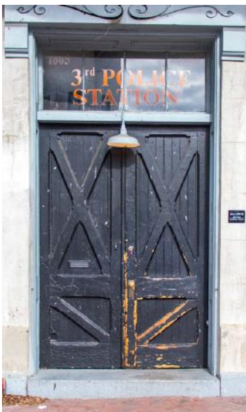
Figure 5. Door 1, first floor entry door.
