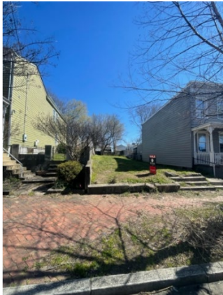
Figure 5. 907 N. 24 th Street, vacant lot. Front retaining wall in poor condition
