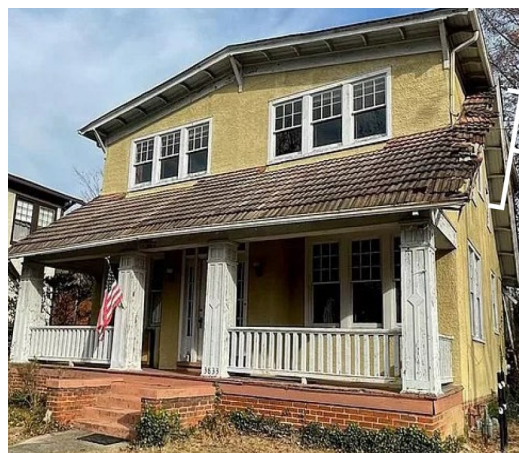
Figure 2. Deteriorated Concrete Tile Roof, 3833 Hermitage Road. Before
