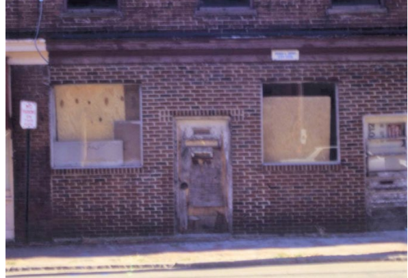
Figure 2. 411 Brook Road, 1997. Storefront infilled with brick. Poor condition. Original materials and configuration have been removed/altered.
