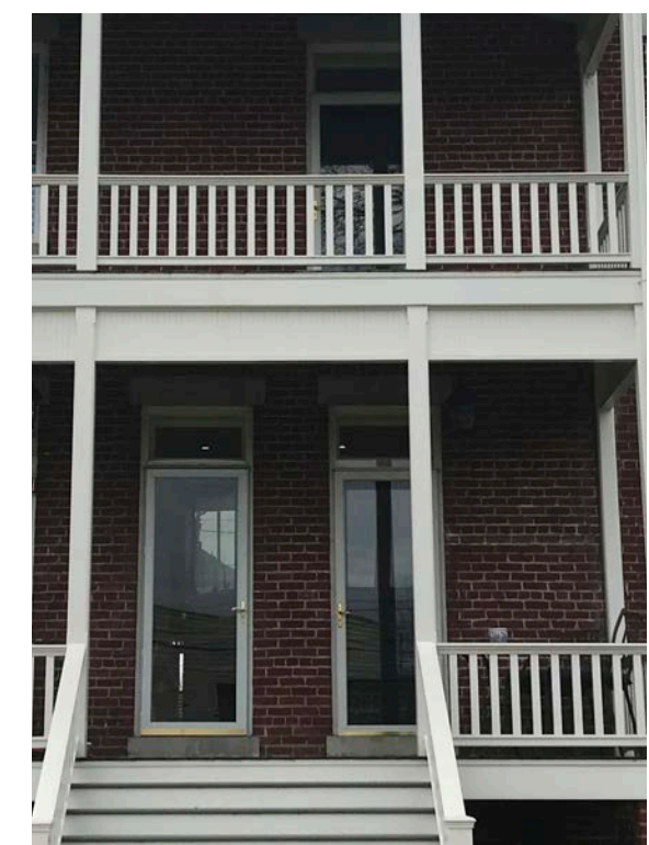
EXISTING REAR DOORS
