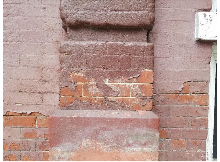
Figure 6. Evidence of original brick color.
