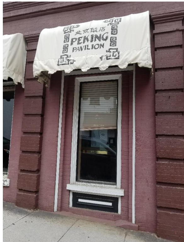
Figure 4. South 13th Street window to become a door.
