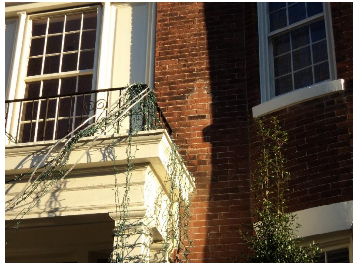
Figure 4. Ghosting of roof balustrade
