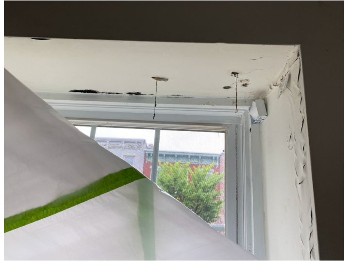
Figure 4. Interior water damage and mold
