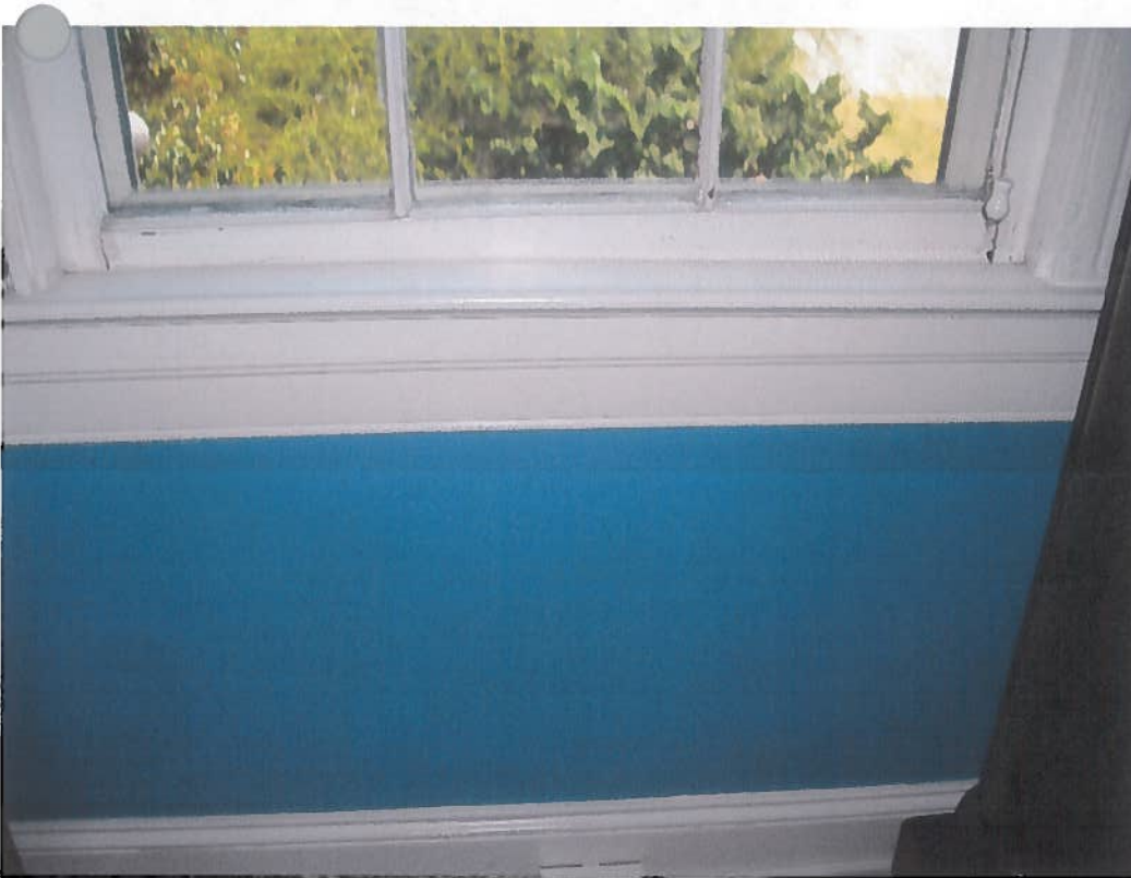
Figure 7: The window sill is level but note the how the window itself is tilted up on the right side.
