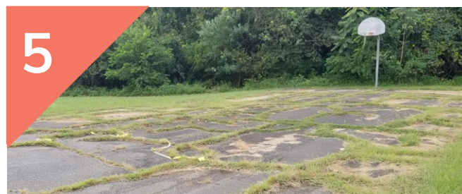
Basketball Court in Briel Park with an overgrown, cracked court.
