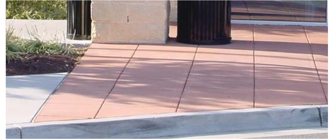
STAINED CONCRETE AT TUCKAHOE LIBRARY
