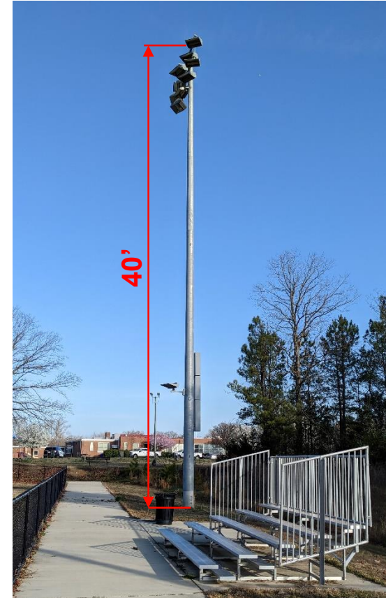
Existing Ball Field Lights
