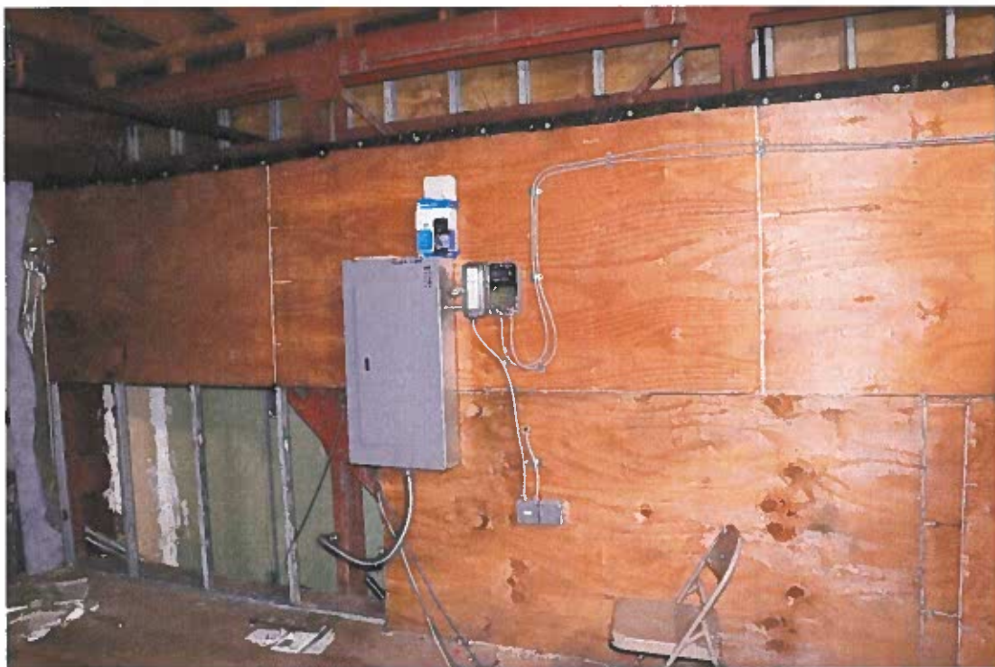
Photo 20. Electrical junction box for illuminated signage (located at base of bell tower), Belgian Building, 11/17/21
