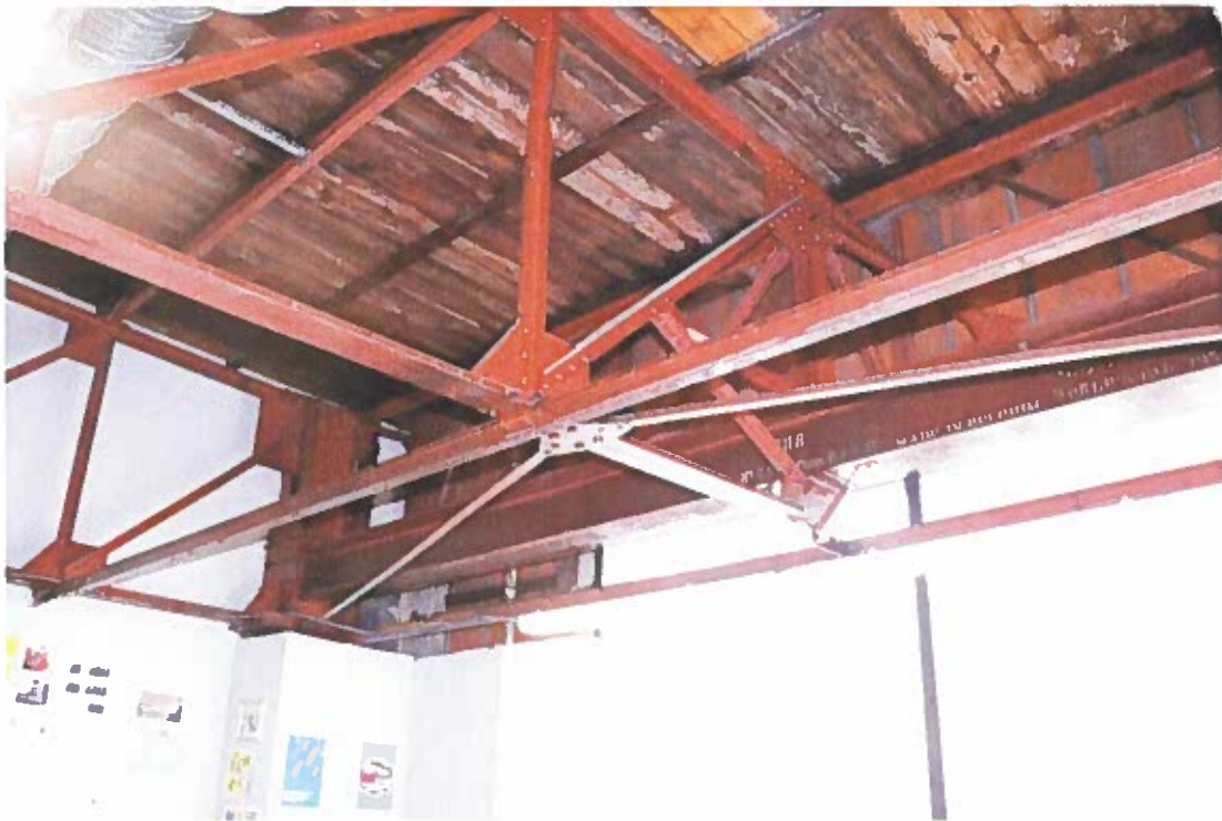
Photo 18. Detail of steel trusses on second floor of arts building, Belgian Building, 11/17/21
