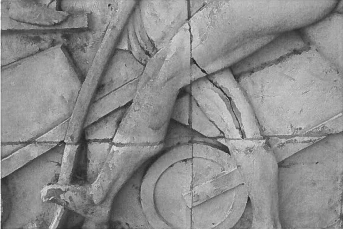
Photo 5. Detail of typical deterioration on bas-relief panel, Belgian Building, 11/17/21
