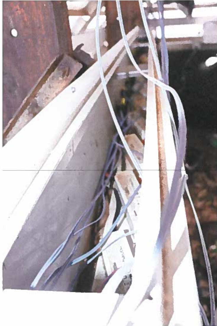
Photo 23. Detail of electrical wiring box located at base of each signage support structure, Belgian Building, 11/17/21
