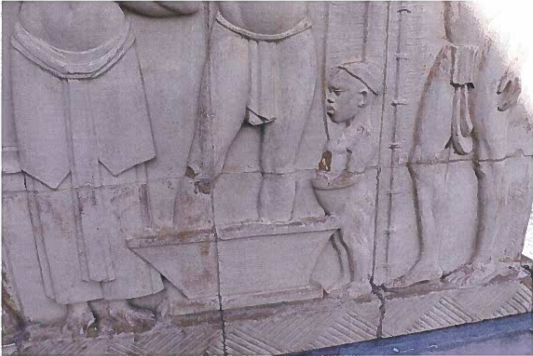
Photo 7. Detail of typical deterioration on bas-relief panel, Belgian Building, 11/17/21
