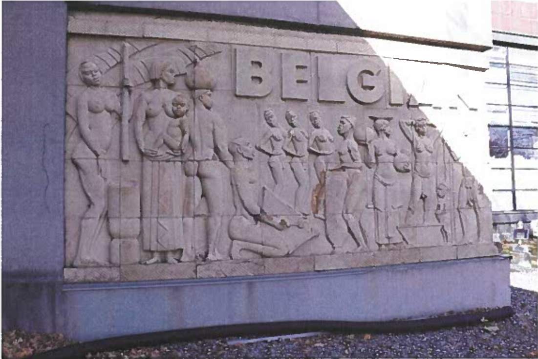
Photo 3. Detail of southeast facing panel on tower base, Belgian Building, 11/17/21
