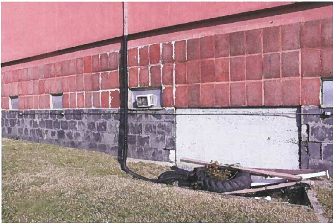
Photo 8. Detail of tile repair on southwest façade of gymnasium building, Belgian Building, 11/17/21
